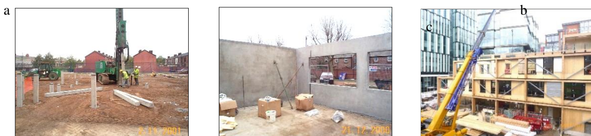
Figure 1 (a) precast concrete piles; (b) precast concrete frame; (c) structural timber frame.
